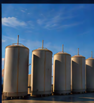
DRY STORAGE / FUEL POOLS
